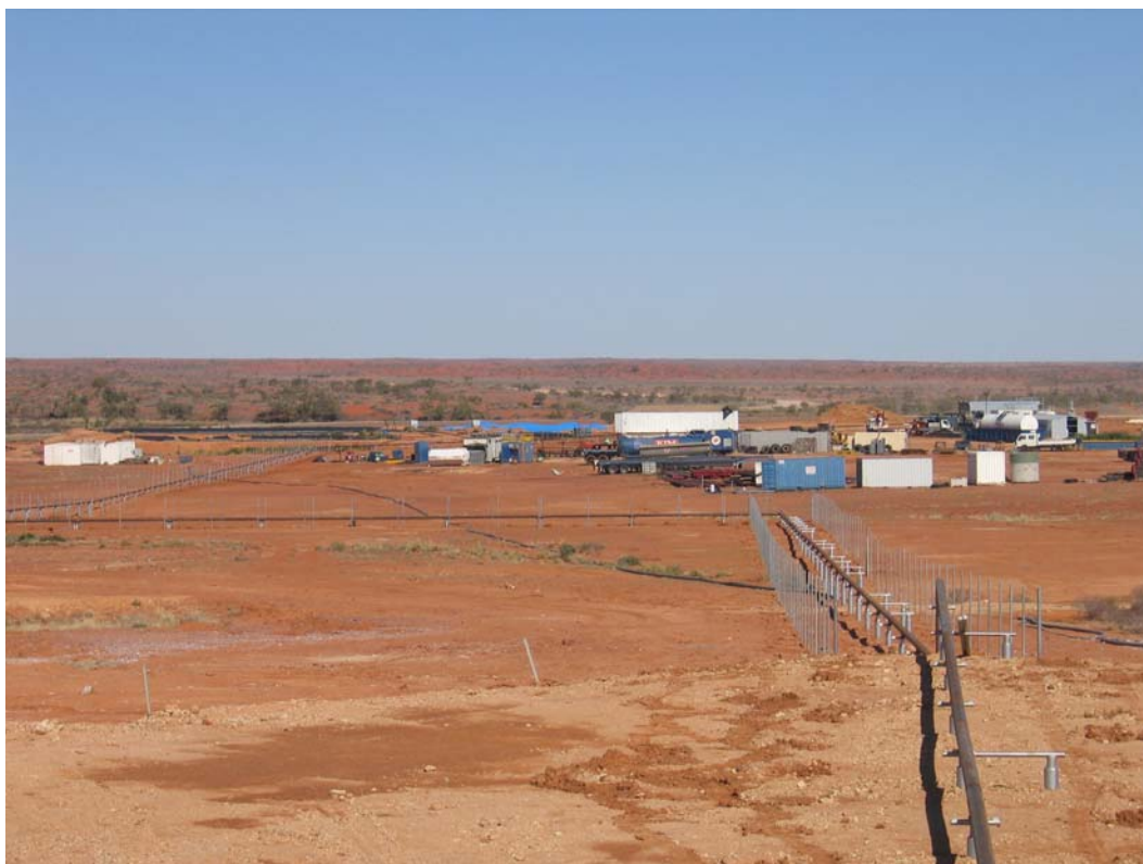
Flow Line looking back from Habanero 3 to Habanero 1
